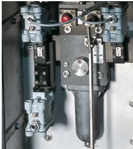
Shown with remote control 0 and SHUT-DOWN in case of power failure
