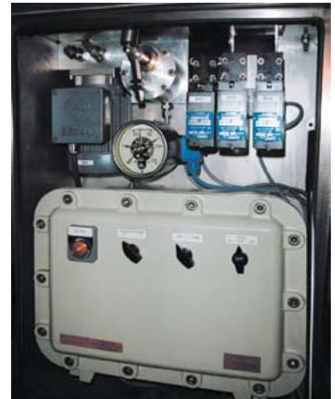
Shown with remote control 0 and SHUT-DOWN travel in case of power failure
